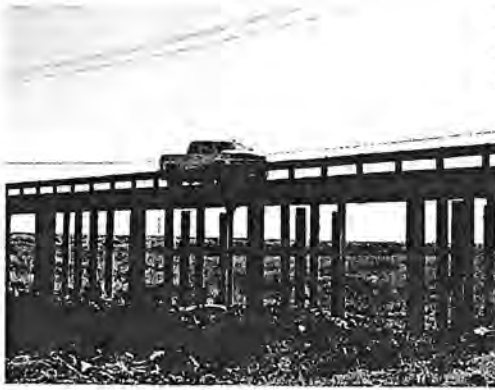
Excessive groundwater pumping caused the land to sink beneath this bridge over the Eastside Bypass between Firebaugh and Madera. Concrete posts that used to support the bridge, sank along with the land and had to be replaced. Lois Henry / SJV Water
