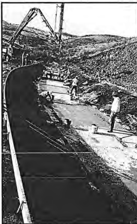
The Kittitas Reclamation District’s South Branch Canal is being alternately lined and piped as is most efficient and otherwise suited for each area. Projects are funded in part by Reclamation grants. Photo courtesy of Kittitas Reclamation District.
