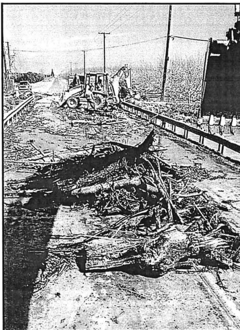
San Joaquin Valley Tom Barcellos and his crew clear debris from under a bridge to keep floodwaters flowing. Photo courtesy of Tom Barcellos.
