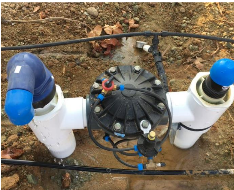
Pressure regulator at the head of a manifold
