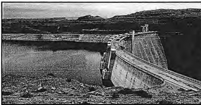
Glen Canyon Dam in Arizona holding back Lake Powell. Photo courtesy of U.S. Bureau of Reclamation.
