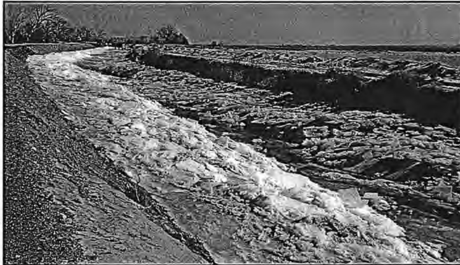
The Truckee Canal (pictured here, with ice) in Nevada's Lahontan Project will receive IIJA funds to line a section of the canal with geomembrane and concrete. Photo source: Bureau of Reclamation
